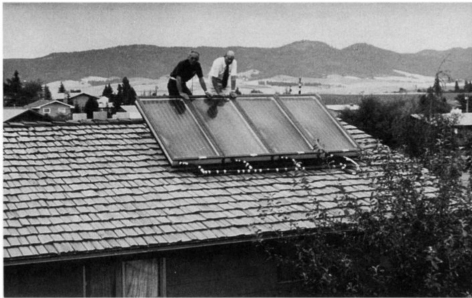
In the energy-conscious era of the 1970s, NASA's operational experience found many new applications. This prototype water heater, warmed by solar cells, was installed on a home in Idaho.
