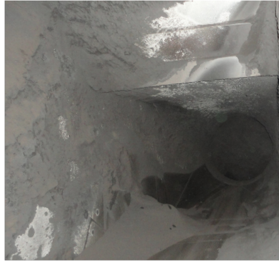
(B) Another photo of material build-up in a chute.
