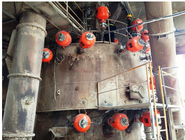
FIGURE 11.18. A photograph showing the installation of multiple (orange) air cannons on a hopper. This figure is from https://www.martin-eng.com/content/product_subcategory/491/air-cannons-products .
