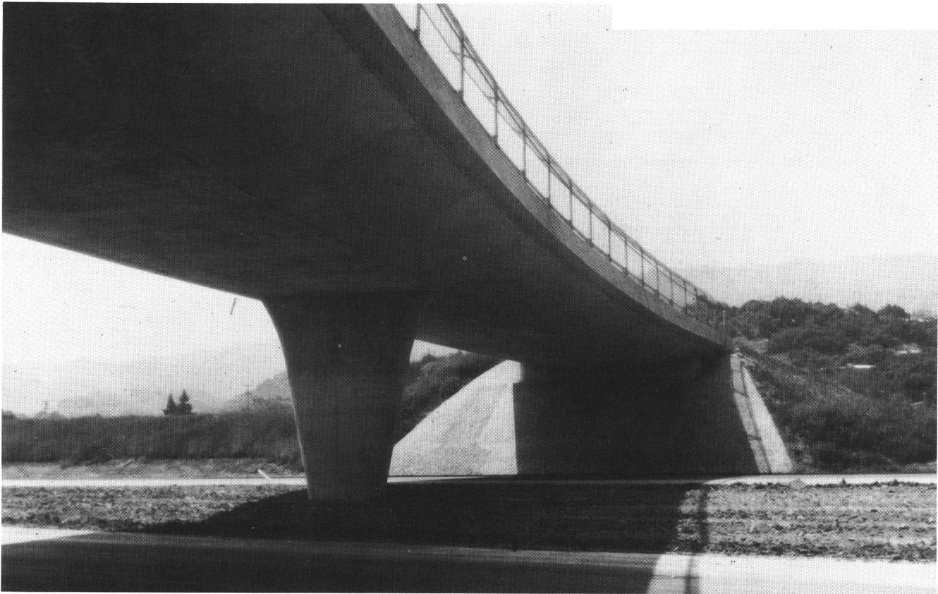
Overcrossing in California with curved alignment and curved soffit (note flared integrated pier and unobstrusive abutments)
