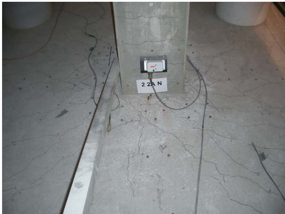
Figure 3-101 Level 2 Column 2A North Final Cracks
