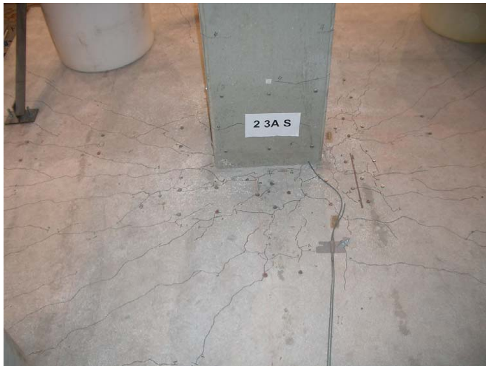
Figure 3-77 Level 2 Column 3A South Final Cracks
