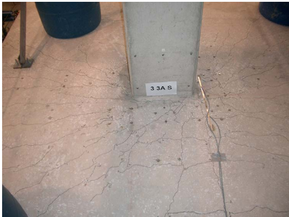
Figure 3-85 Level 3 Column 3A South Final Cracks
