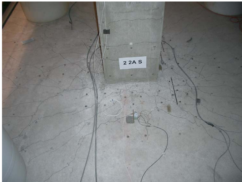
Figure 3-75 Level 2 Column 2A South Final Cracks
