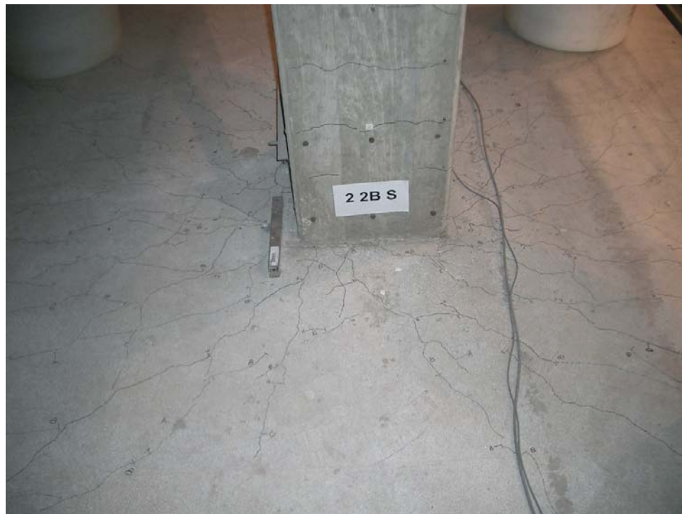
Figure 3-79 Level 2 Column 2B South Final Cracks
