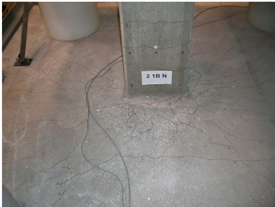
Figure 3-103 Level 2 Column 1B North Final Cracks
