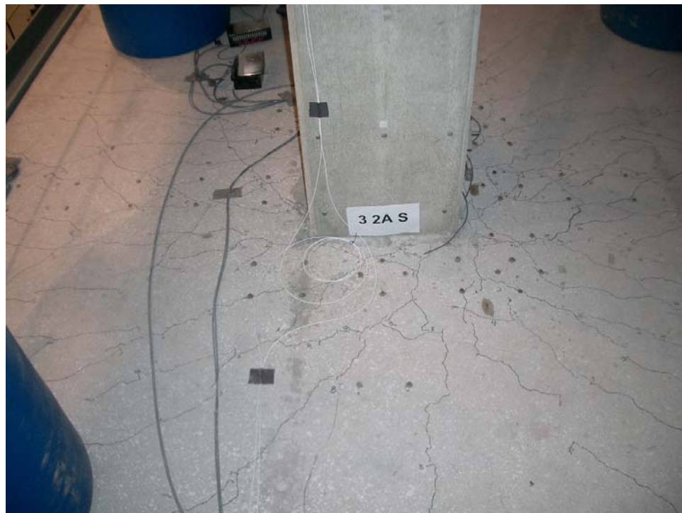
Figure 3-83 Level 3 Column 2A South Final Cracks
