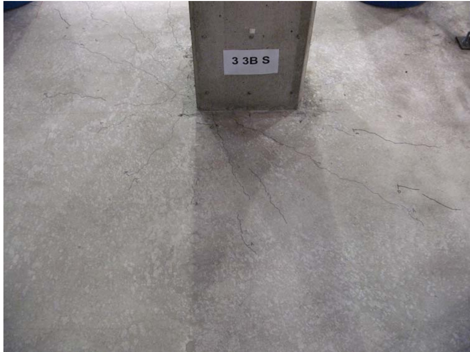
Figure 3-88 Level 3 Column 3B South Initial Cracks
