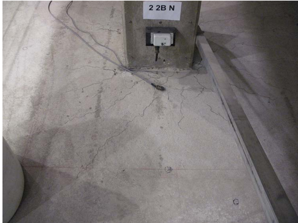
Figure 3-104 Level 2 Column 2B North Initial Cracks
