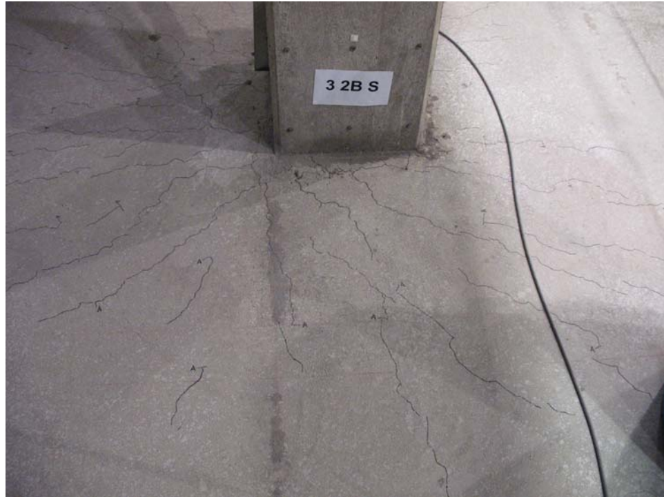
Figure 3-86 Level 3 Column 2B South Initial Cracks
