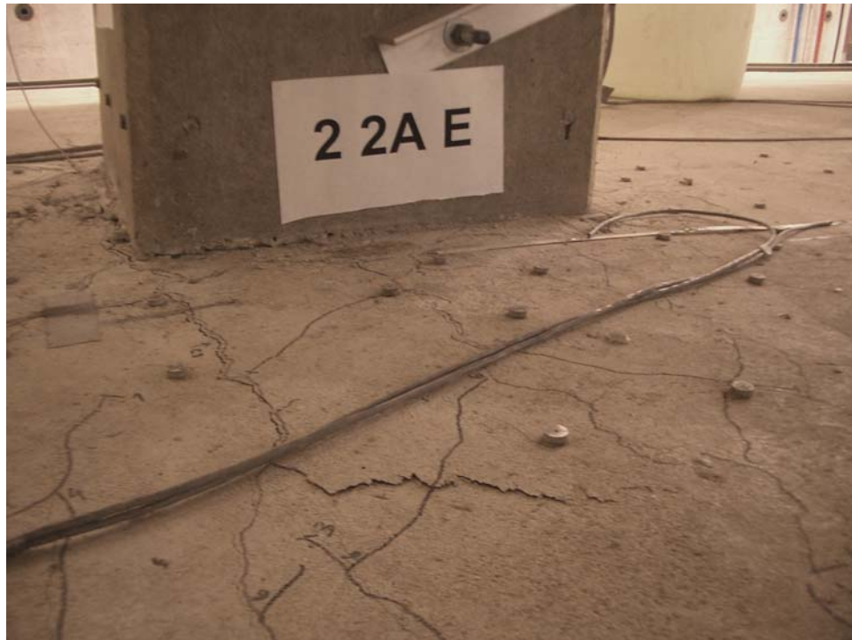
Figure 3-22 Vertical Slab Separation (North 3% Roof Drift Ratio)
