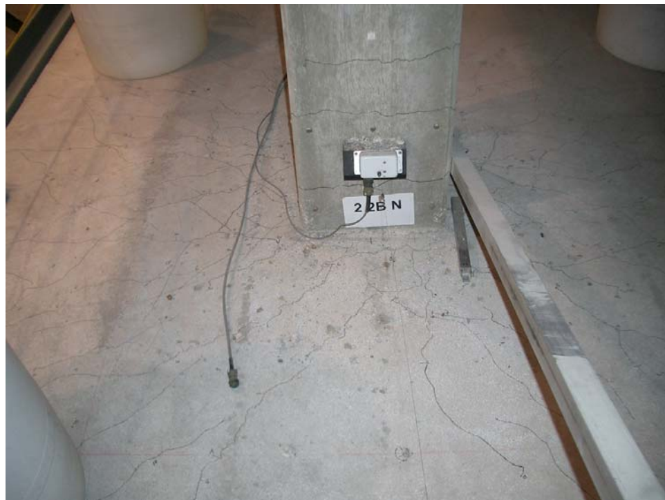
Figure 3-105 Level 2 Column 2B North Final Cracks
