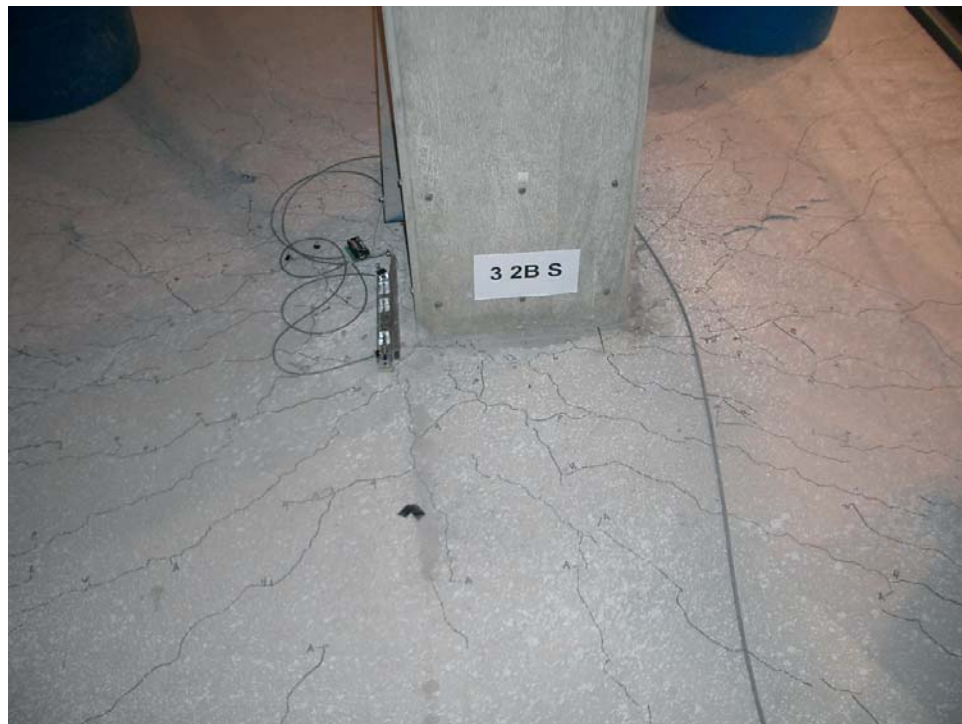
Figure 3-87 Level 3 Column 2B South Final Cracks
