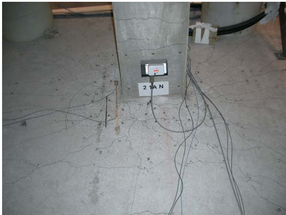
Figure 3-99 Level 2 Column 1A North Final Cracks
