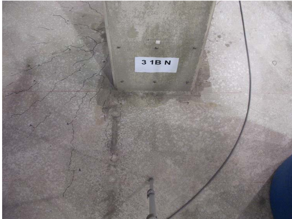
Figure 3-110 Level 3 Column 1B North Initial Cracks
