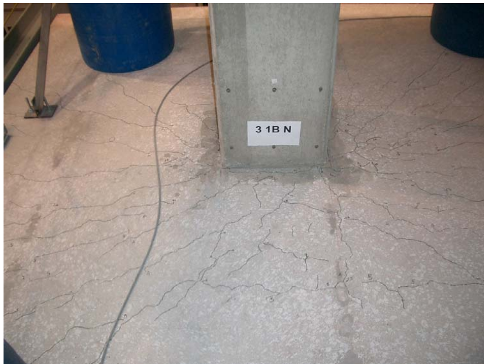
Figure 3-111 Level 3 Column 1B North Final Cracks
