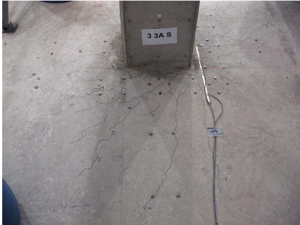
Figure 3-84 Level 3 Column 3A South Initial Cracks
