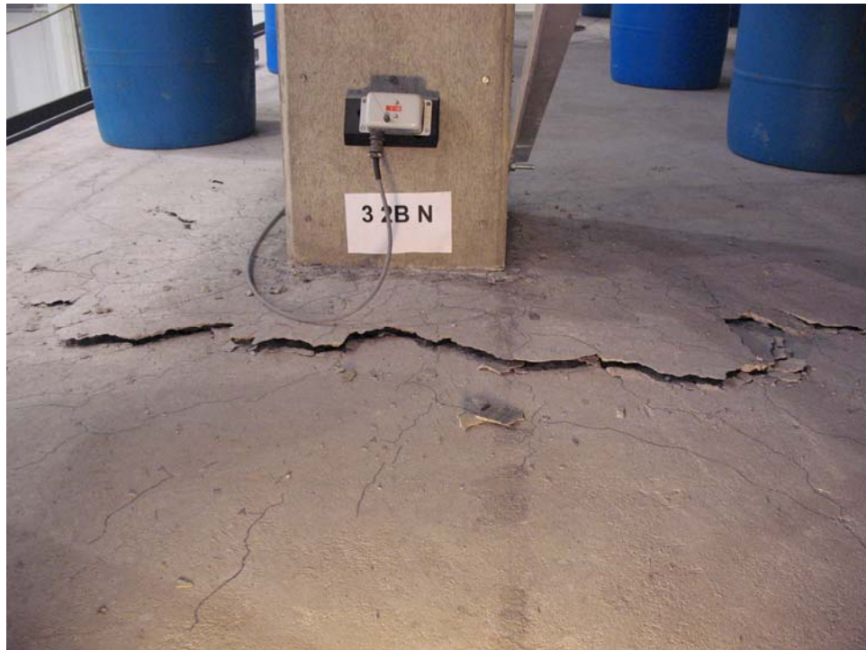
Figure 3-14 Slab-Column Connection Failure
