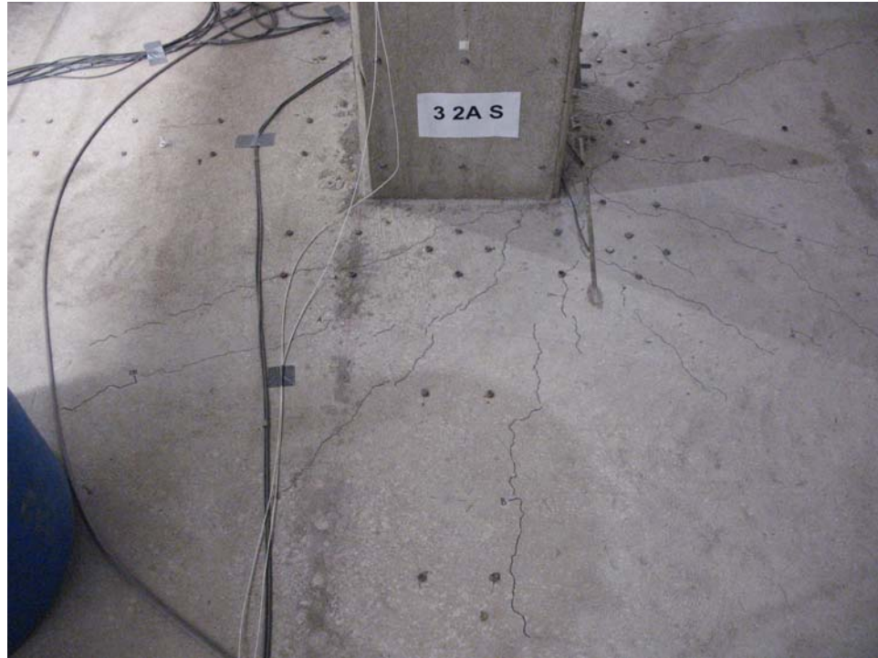
Figure 3-82 Level 3 Column 2A South Initial Cracks
