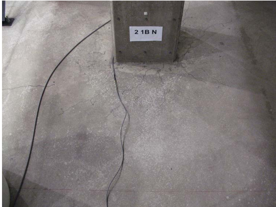
Figure 3-102 Level 2 Column 1B North Initial Cracks
