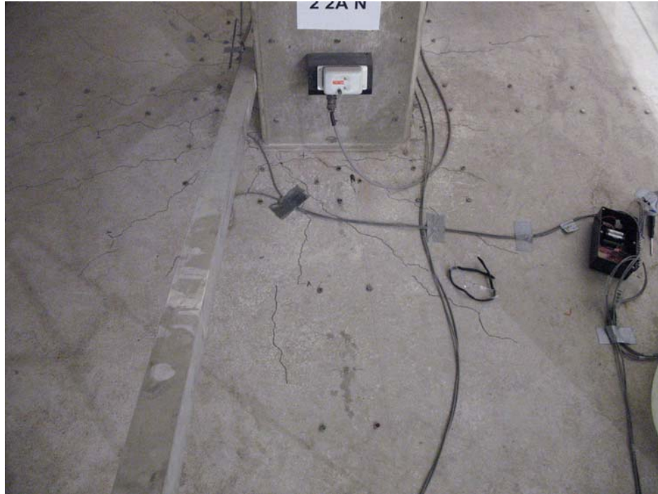
Figure 3-100 Level 2 Column 2A North Initial Cracks
