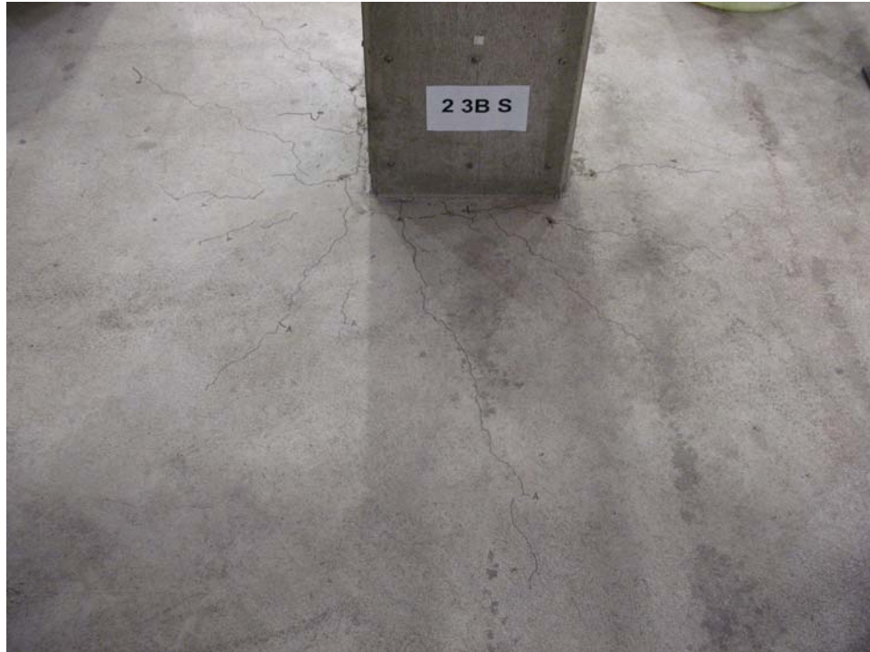
Figure 3-80 Level 2 Column 3B South Initial Cracks
