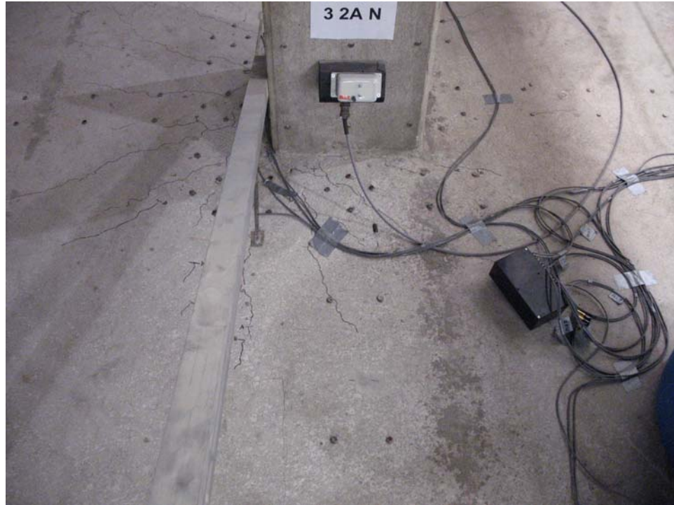
Figure 3-108 Level 3 Column 2A North Initial Cracks
