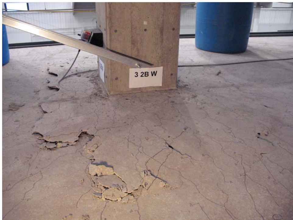
Figure 3-15 Slab Column Connection Failure
