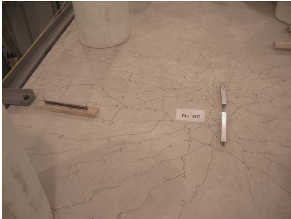
Figure 3-121 Roof Column 2B North Final Cracks
