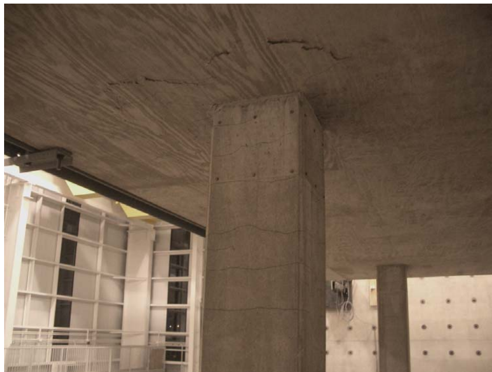
Figure 3-23 Vertical Slab Separation (South 3% Roof Drift Ratio, Column 3-2B-N)
