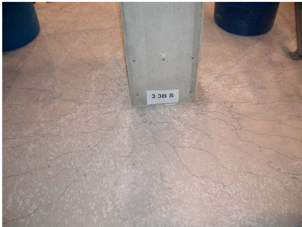
Figure 3-89 Level 3 Column 3B South Final Cracks
