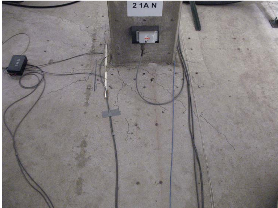
Figure 3-98 Level 2 Column 1A North Initial Cracks
