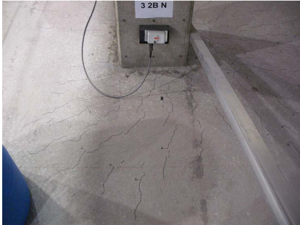
Figure 3-112 Level 3 Column 2B North Initial Cracks
