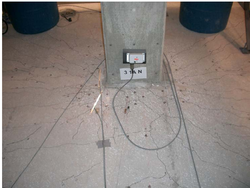
Figure 3-107 Level 3 Column 1A North Final Cracks
