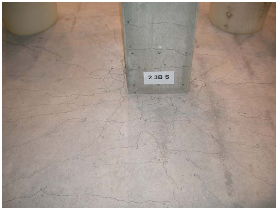
Figure 3-81 Level 2 Column 3B South Final Cracks
