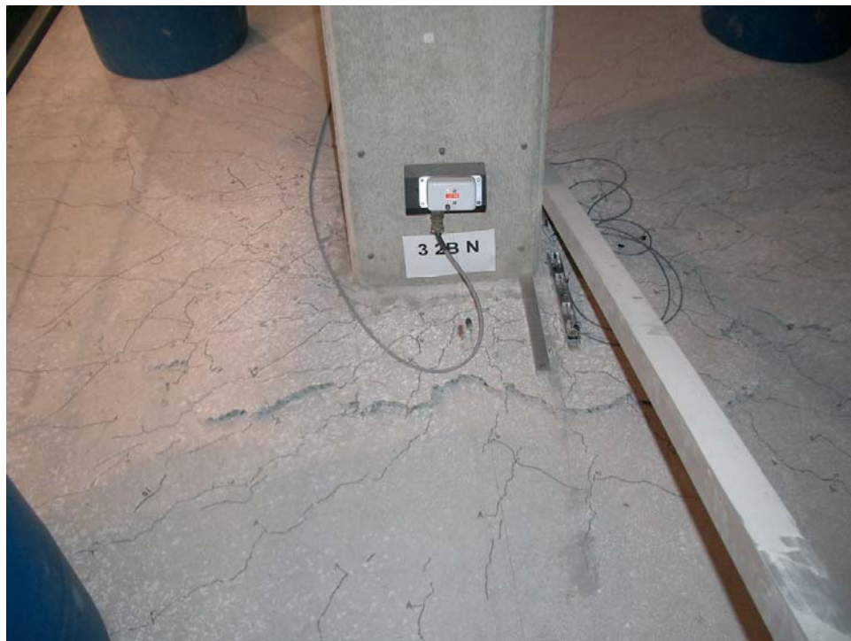
Figure 3-113 Level 3 Column 2B North Final Cracks
