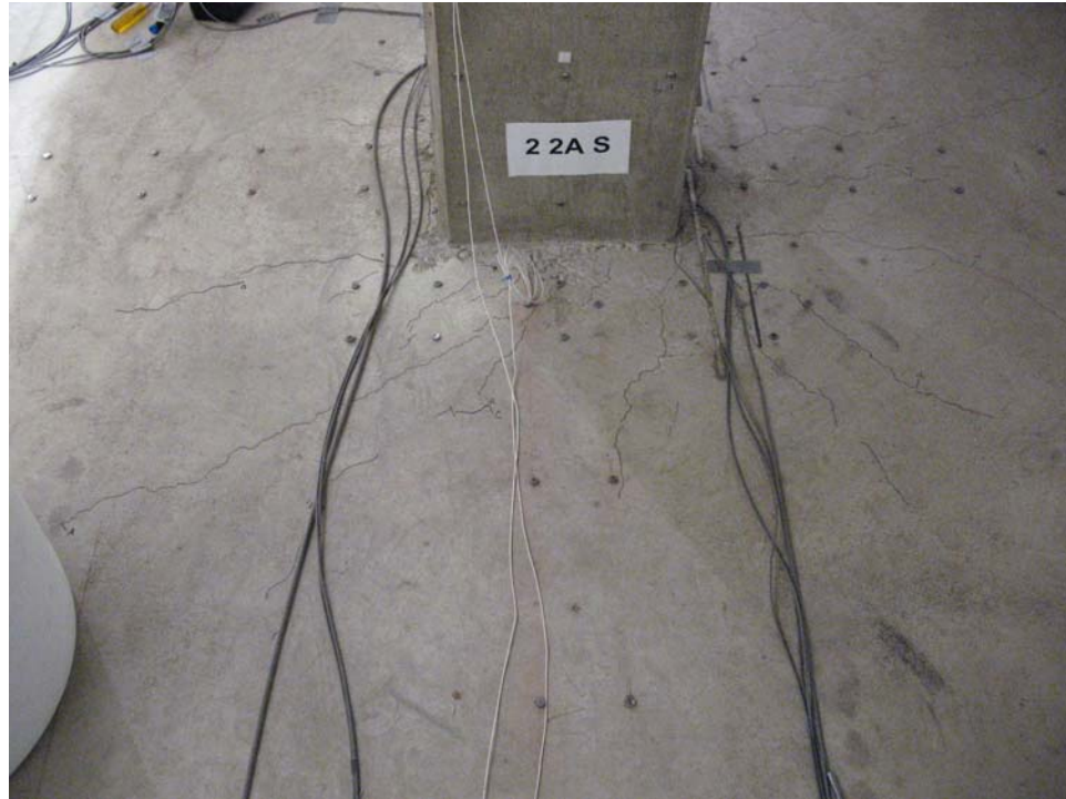
Figure 3-74 Level 2 Column 2A South Initial Cracks
