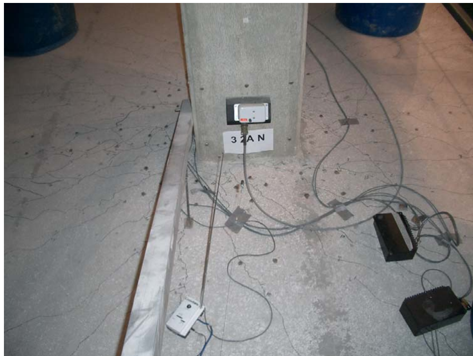
Figure 3-109 Level 3 Column 2A North Final Cracks
