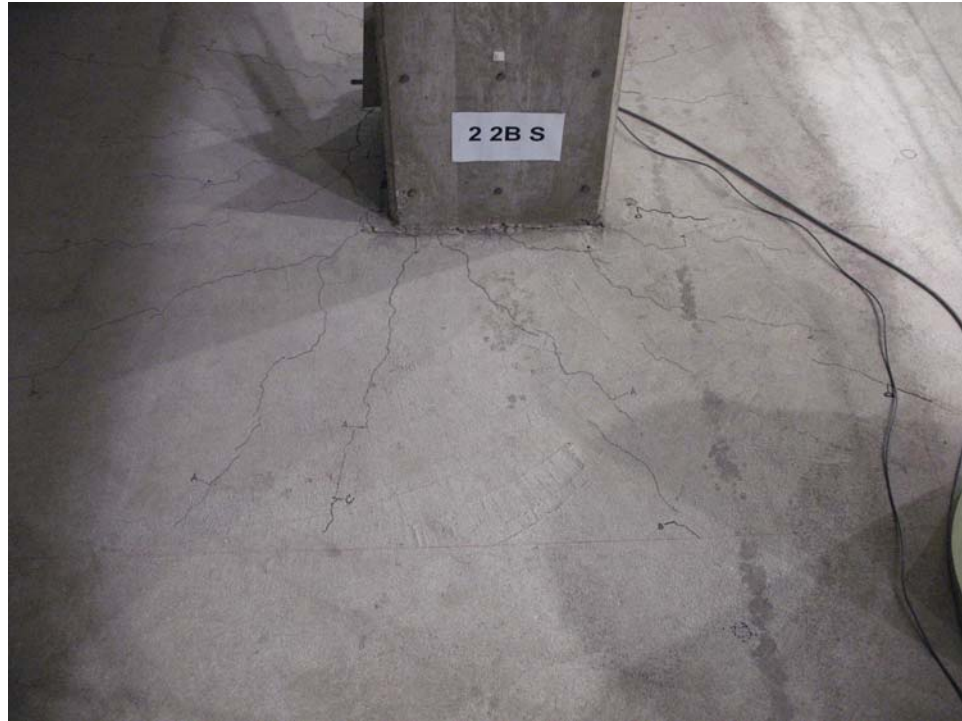
Figure 3-78 Level 2 Column 2B South Initial Cracks
