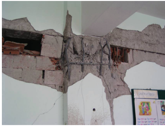
Figure 10. A captive column in Building C14-01 created by the crushing of the corner regions of infill walls.
