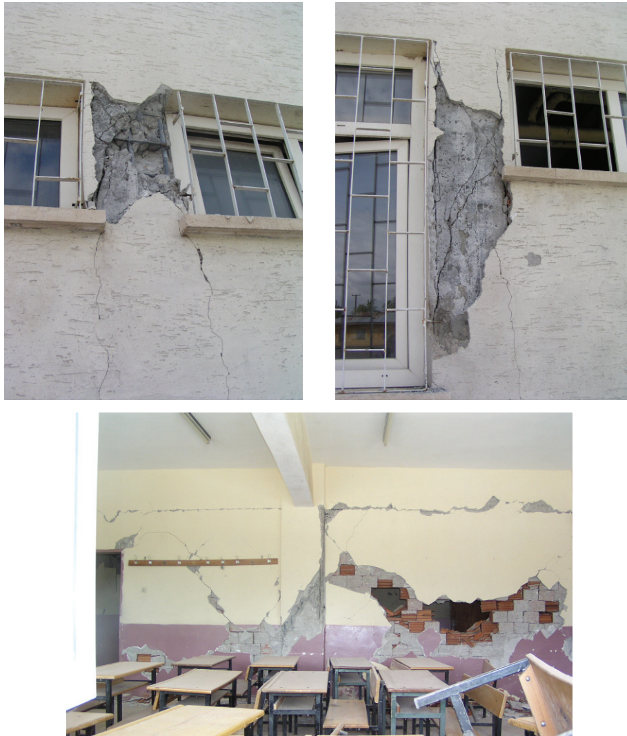
Figure 2. Examples of severe column damage.
