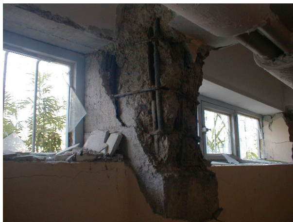
Figure 14. A failed captive column in the basement of Building D02.
