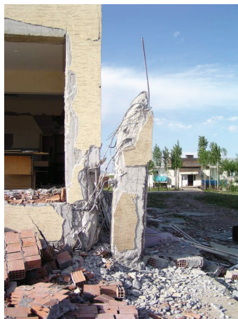
Figure 9. The remains of the corner column of the ground floor of the building shown in Fig. 7 (Building C13-09). The corner column failed in shear.
