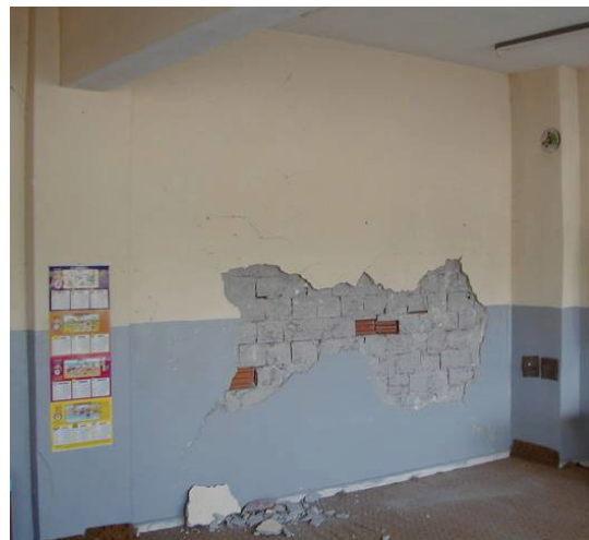
Figure 4. A moderately-damaged masonry wall.
