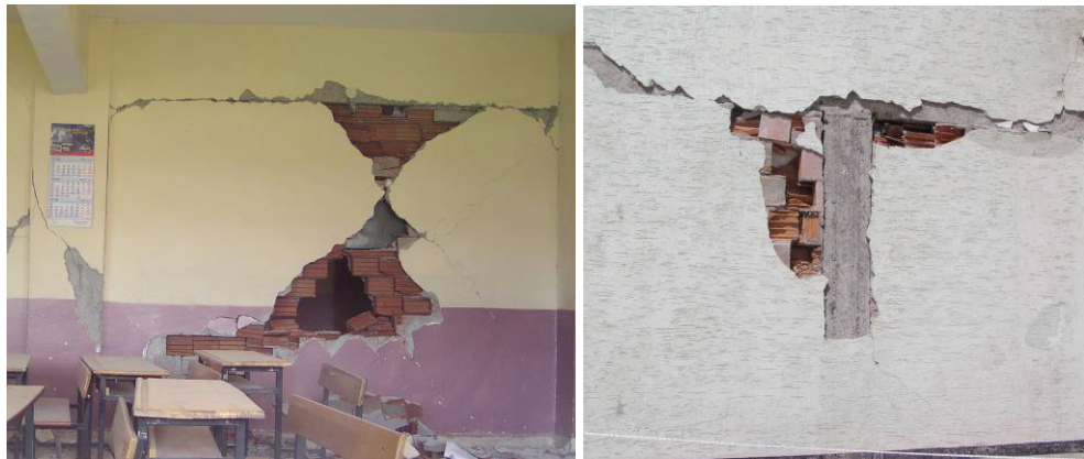
Figure 3. Examples of severe masonry-wall damage.
