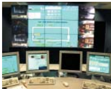
Planned State-of-the-Art Control Room for VKF
