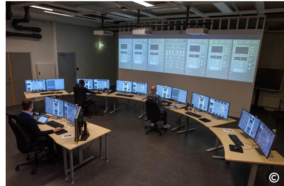
IFE HAMMLAB SMR Control Room Simulator
