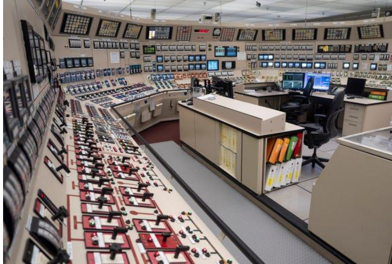
Watts Bar Control Room Simulator
