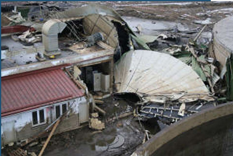
Damage in an AD incident
