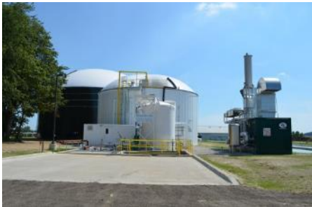
CSTR system (2000 m 3 , 0.4 MW)
