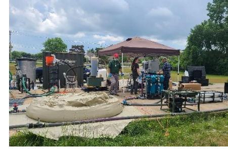
Pilot water and energy testing site
