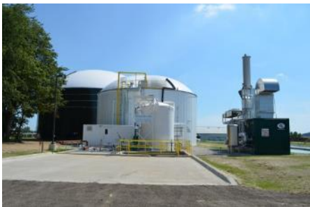
CSTR system (2000 m 3 , 0.5 MW)
