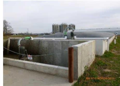
A plug-flow digester (1,000 m 3 )
