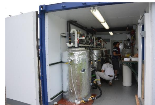
The container waste utilization unit
