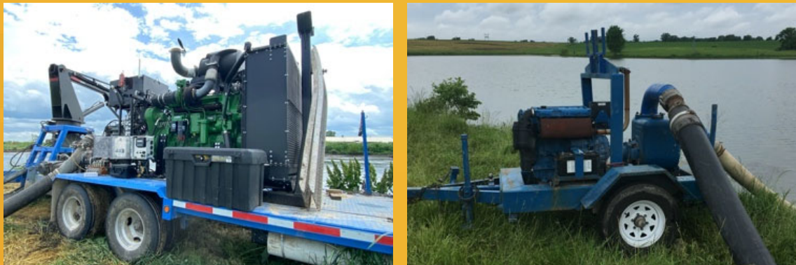
Primary lagoon pump (trailer mounted, left) and dilution pump (right).
