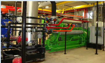
Generates 1.06 MW of electricity
