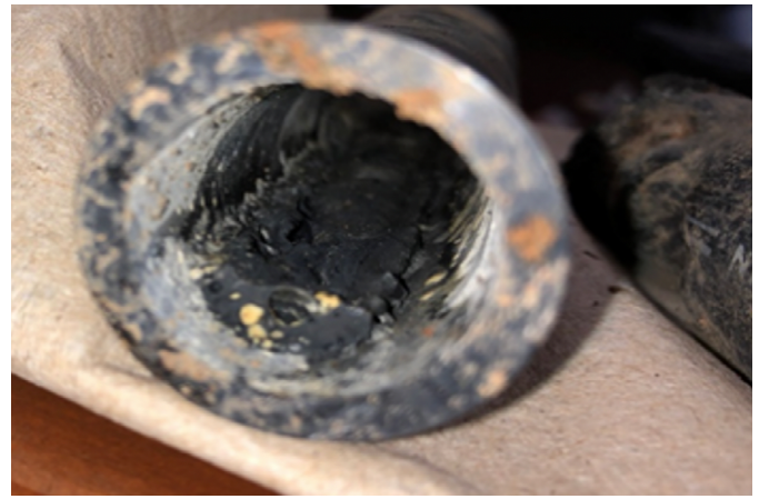
Degraded plastic pipe following wildfire
