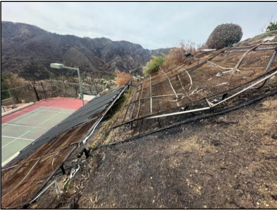
Solar and battery infrastructure
