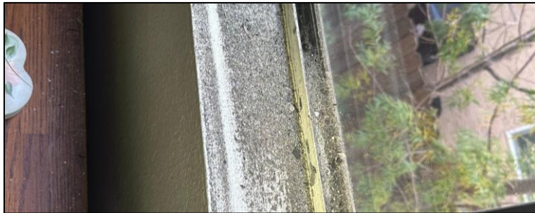
Surface dust on windowsills and throughout interior
