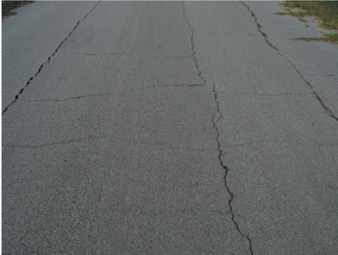
Shrinkage Cracking Resulting from Problems with Cement-Treated Base (internet image)
