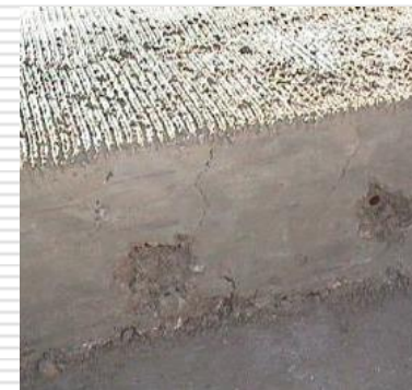
Examples of plastic shrinkage cracking (source Internet)
