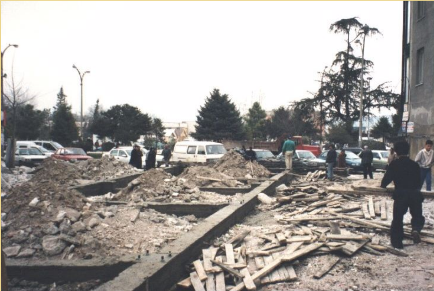
Adapazari. Typical Foundation
