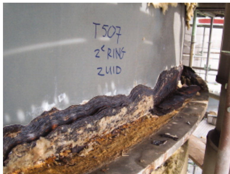
Figure 10. Damage due to uncoated metal can be seen. Such damage can be prevented by applying anti-resistant sprays to metals before their service life begins. 4
