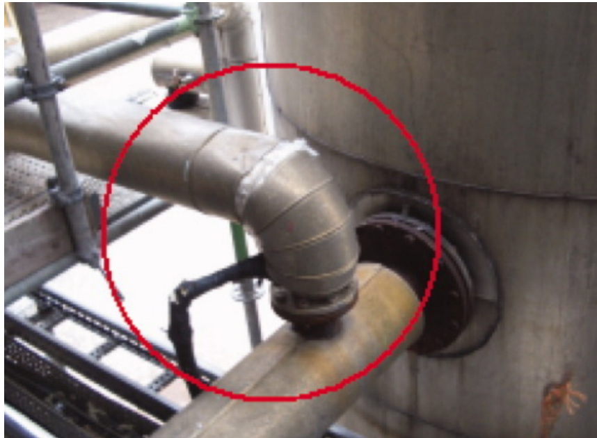
Figure 4. The damage in the elbow is shown. More frequent inspections could have caught this before it turned into a serious incident. 4
