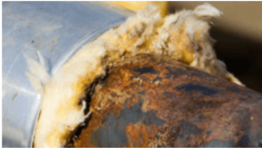
Figure 2. Corrosion under the insulation of a pipe. Note the relative lack of corrosion on the exterior metal cladding compared to the inner pipe. 2
