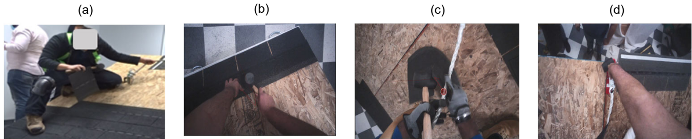
Unsafe behavior: (a) Sitting close to roof edge; (b) Hammer too close to finger; (c) Poor hand coordination; d) Hammer for support at roof tip
