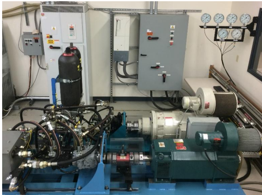
Fig. 20: Blended hybrid hardware-in-the-loop test rig
