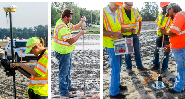
ABOVE Left: GPS Testing (primary method); Middle: DCP Testing (primary method); Right: LWD Testing (secondary method)
