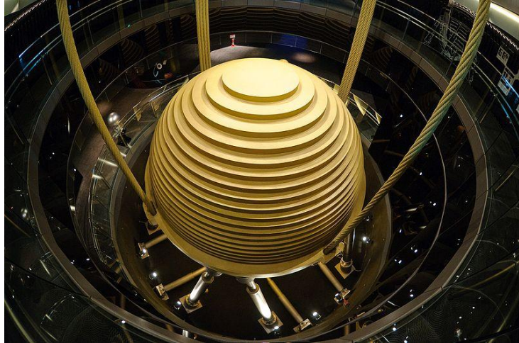
Figure 1.5: TMD installed in Taipei 101 in Taiwan
