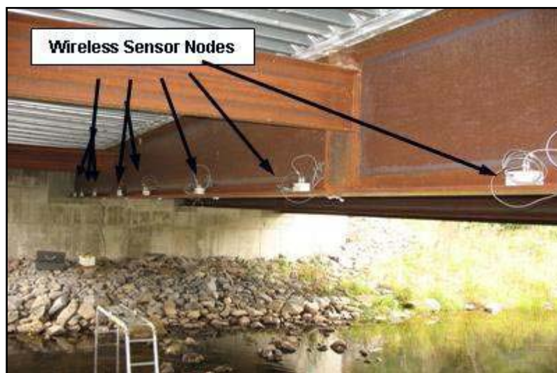
Figure 1.1 Wireless sensor nodes deployed on one of the beam girders (after Gangone et al, 2007)
