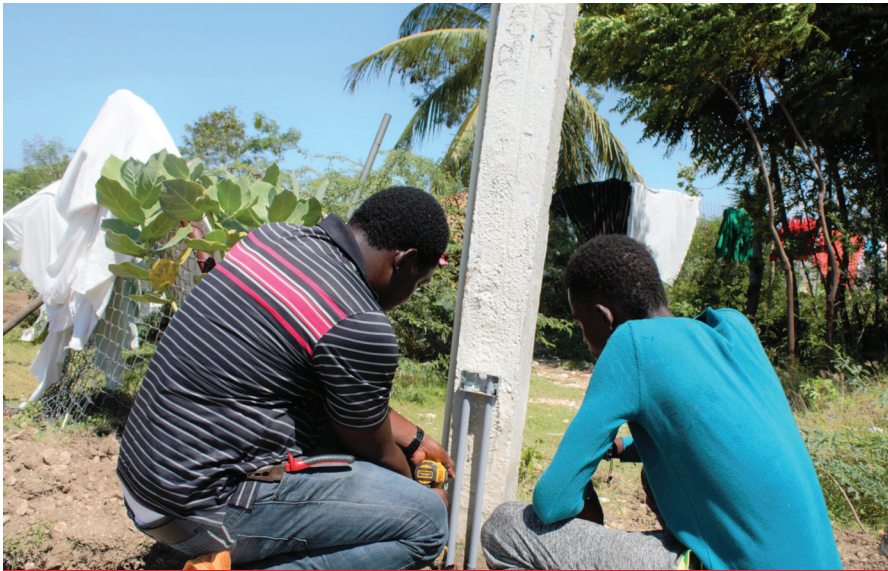
An electrician professor installs lights in the Imagine Missions compound to provide better security.
