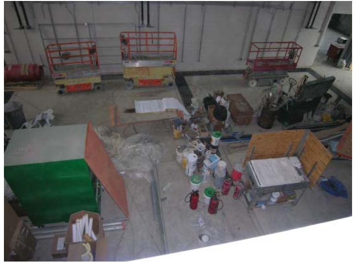
A look into the high bay flexible lab space from the second floor offices.
