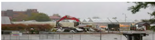
19 th October, 2011 – Demolition of the former Grounds Services' sheds and greenhouse. Picture is facing east. In the background are the greenhouses behind Lily Hall of Life Sciences. (This and all photos on this page are by Gilbert Gordon, Head of Herrick Laboratories Technical Services)
