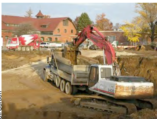
8 th November, 2011 – Hauling away dirt from the big hole getting ready to do the basement foundations. Picture facing northwest with the current Herrick Labs. building in the background.
