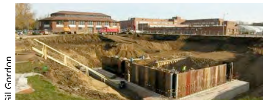
11 th November, 2011 – Wooden forms in place for pouring of the basement walls. The photograph is facing north east with the former Grounds Pavilion in the background.
