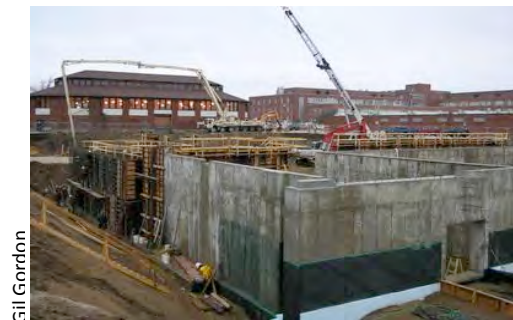
By December 15, 2011 poured walls were visible and part of the basement was waterproofed—a big change since the end of October.
