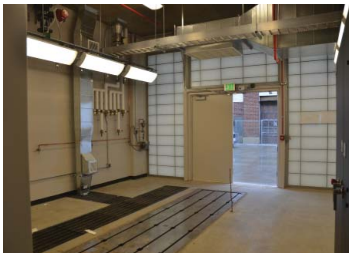
One of 4 engine test cells
