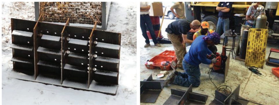
Figure 4.19 (Left) Example of used mockup, (Right) Performance testing of a contractor prior to implementation of a repair project.
