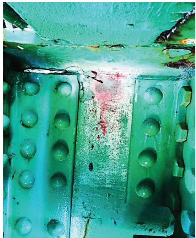
Figure 6.18 Results of PT revealing extent of crack.
