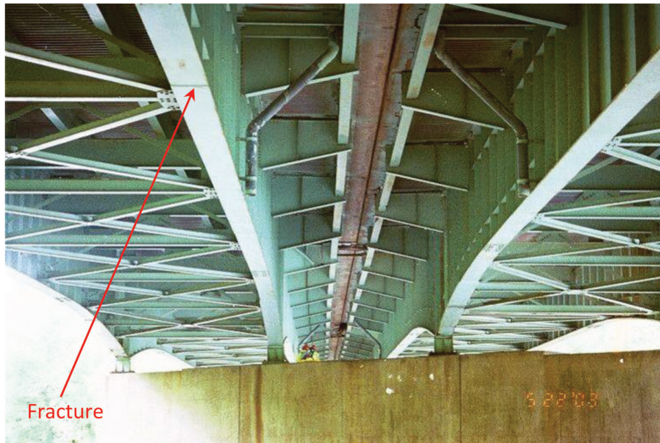
Figure 7.1 US 422 Bridge fracture discovered in 2003 during retrofitting.
