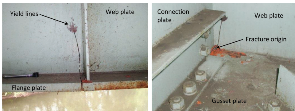
Figure 7.2 US 422 Bridge fracture that arrested in the web.
