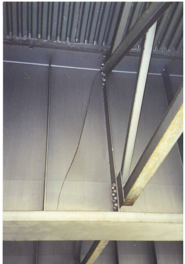
Figure 7.32 Fracture initiated at stiffener in negative moment region (Photograph courtesy of Y. Edward Zhou).
