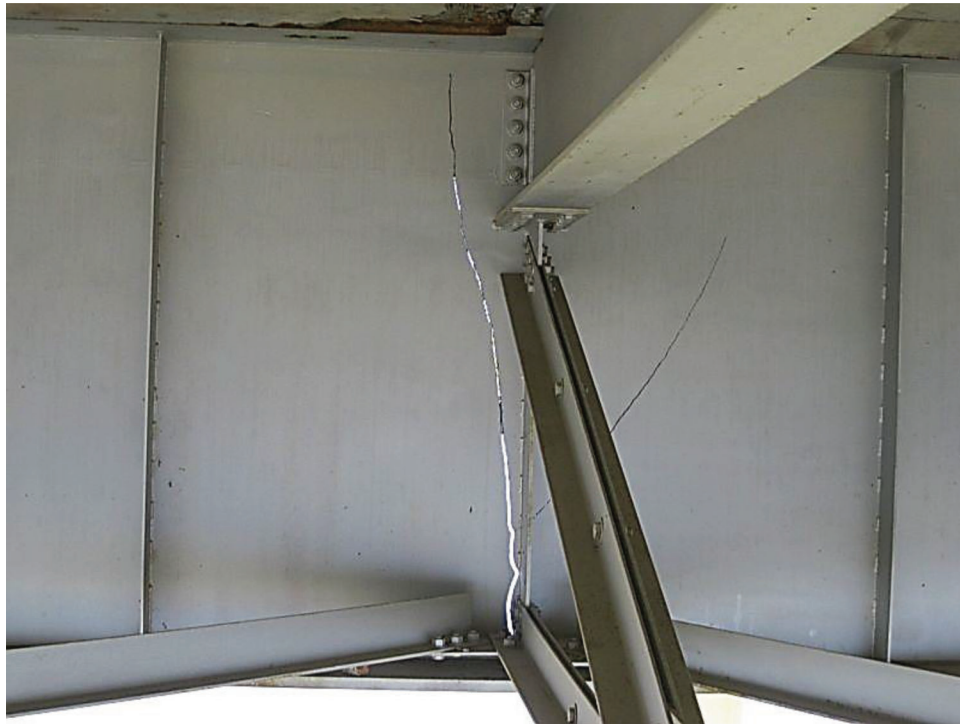
Figure 7.14 Diefenbaker Bridge fracture originated at CIF detail.
