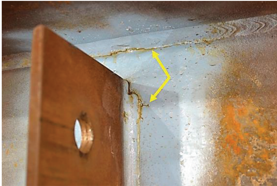
Figure 6.3 Example of web gap cracking resulting from distortion.
