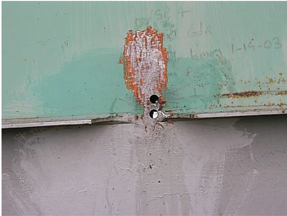
Figure 7.26 Longitudinal stiffener core retrofit showing drilled holes in the web plate for crack arrest (Photograph courtesy of Kansas DOT).
