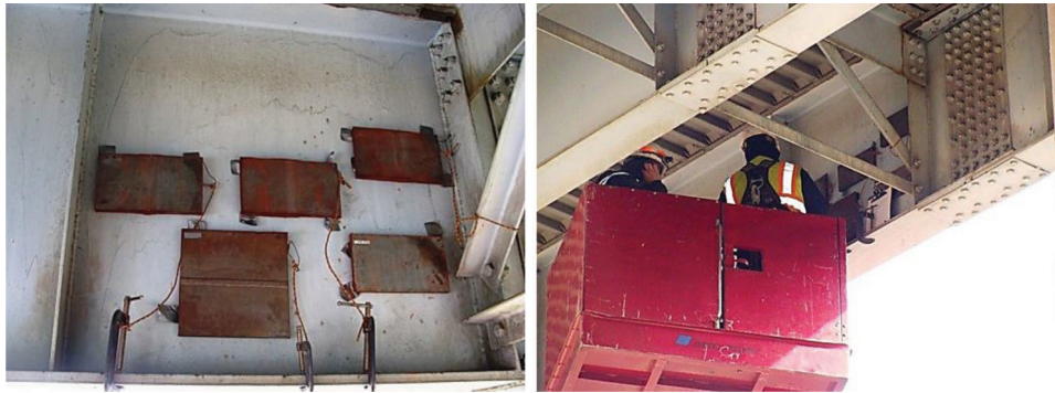
Figure 4.20 (Left) Welded steel test specimen hung on a bridge, (Right) Performance testing of an inspector prior to beginning NDT on bridge welds.
