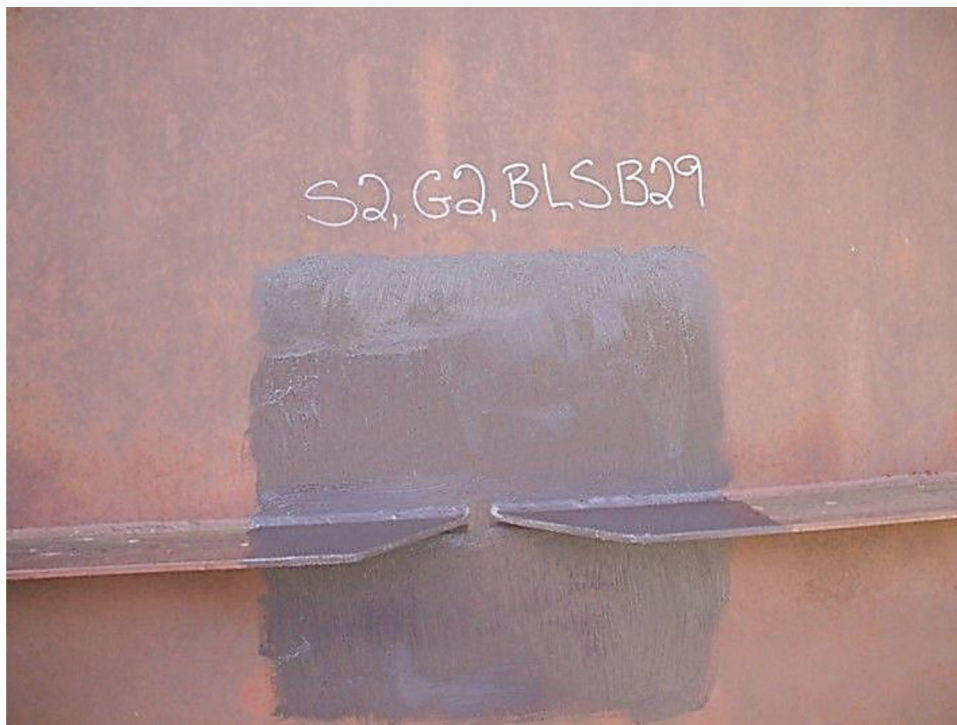
Figure 7.25 Alternate version of the longitudinal stiffener core retrofit with the stiffeners plates cut back in addition to the drilled hole.
