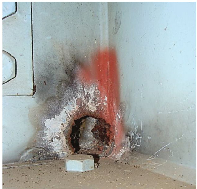
Figure 5.34 Poor quality flame-cut hole that is prone to fatigue and fracture.
