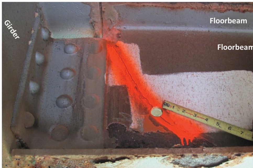
Figure 5.9 Example of load-induced crack at floorbeam cope (Photograph courtesy of Oklahoma DOT).
