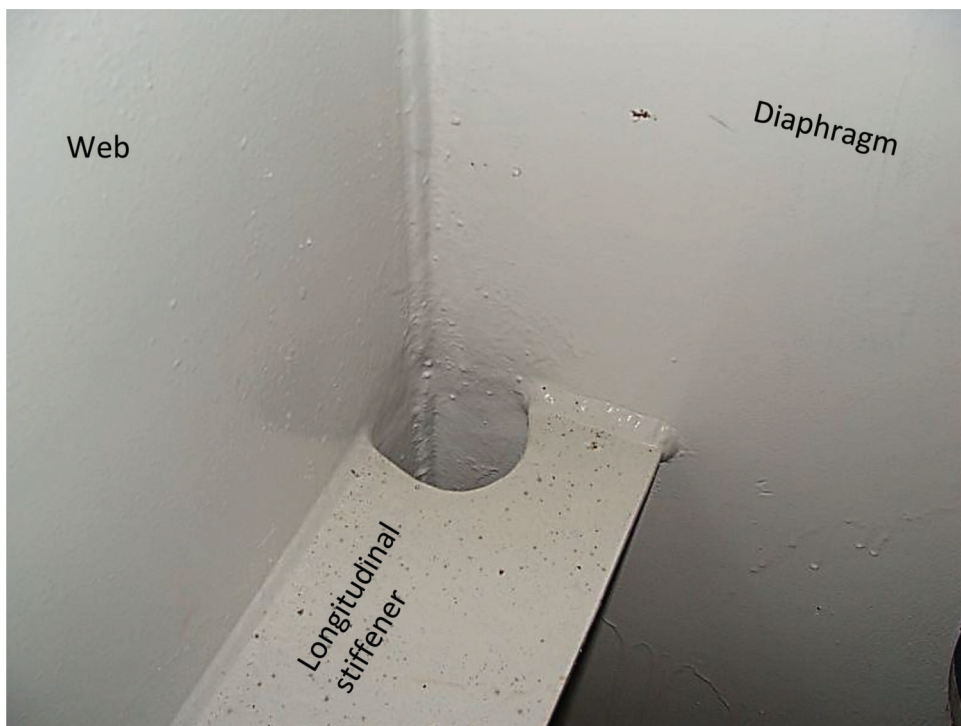
Figure 7.19 Hoan Bridge longitudinal stiffener CIF retrofit.
