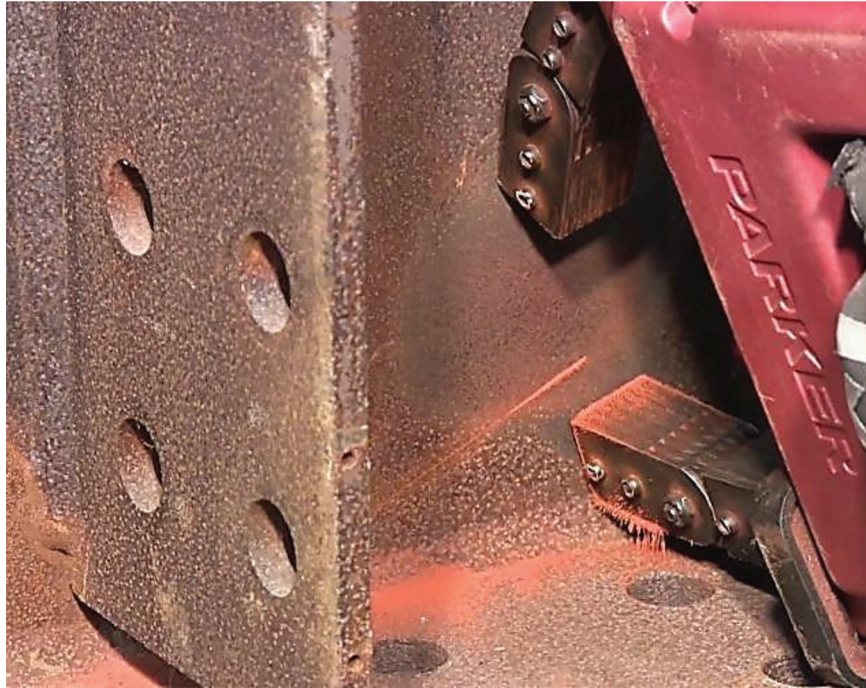
Figure 4.7 Magnetic Particle Test performed before drilling crack arrest hole in order to locate the crack tip.
