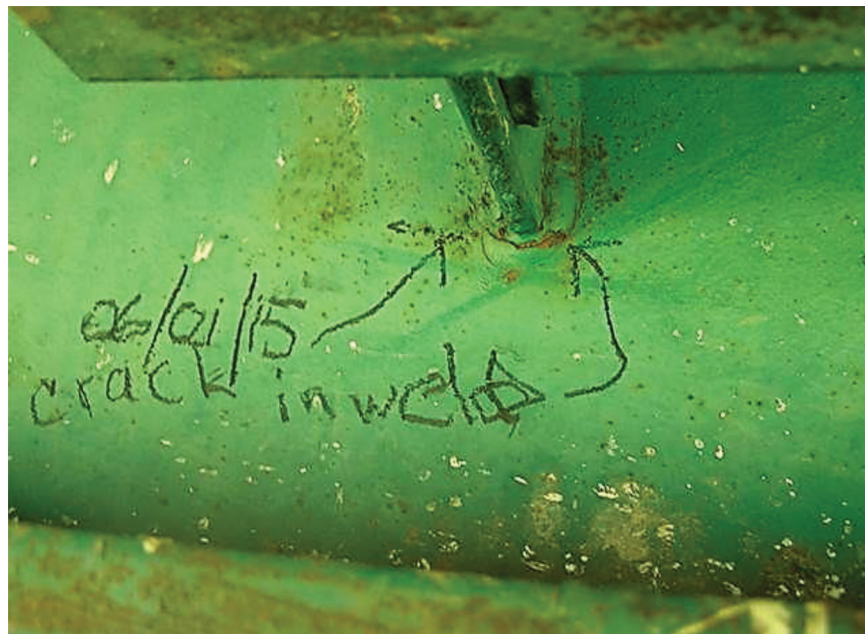
Figure 4.22 Distortion-induced fatigue crack growing out of the throat of the weld.
