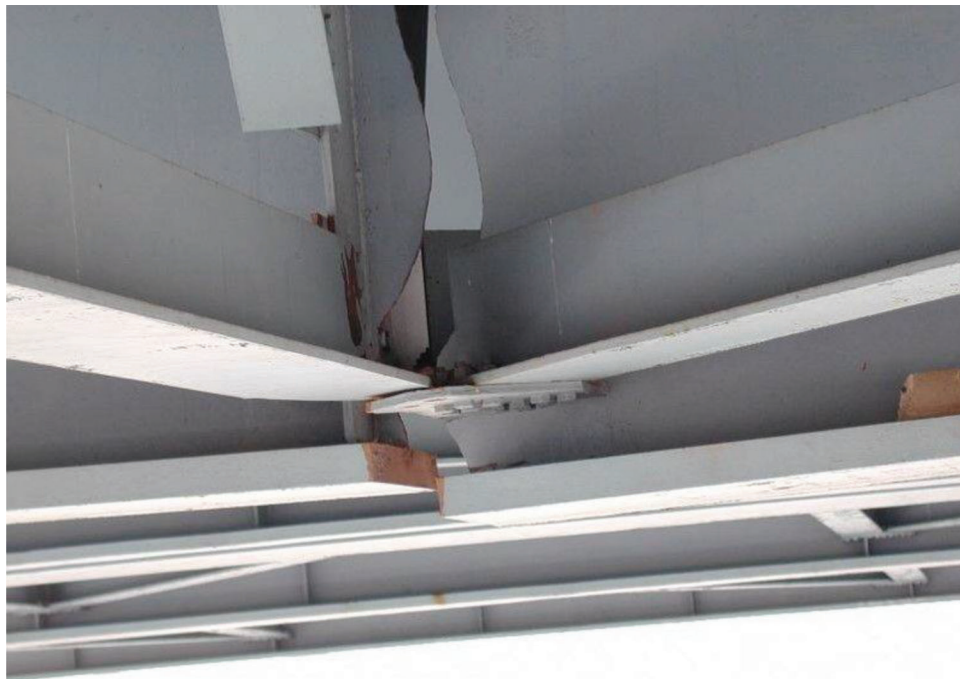
Figure 7.6 Hoan Bridge fracture showing the gusset detail of the interior girder.
