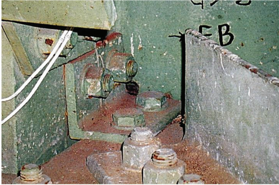
Figure 6.6 Insufficiently stiff splice angle shown installed on gusset-connection plate web gap.
