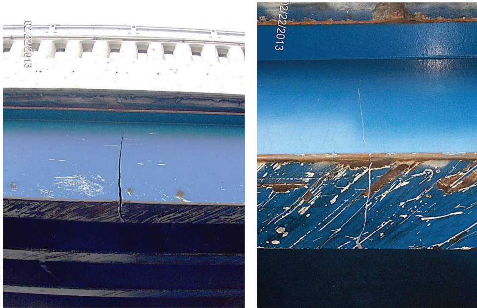
Figure 5.47 Fractures on the same girder resulting from a singled impact event.
