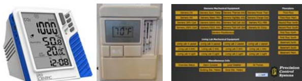
Data logger, thermostat and building automation system
