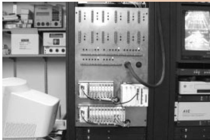
Video and signal status panels
