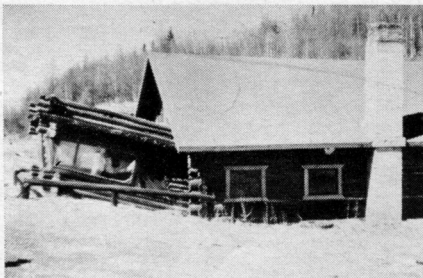
ALASKA HOUSE SINKING INTO PERMAFROST Where a thaw just makes matters worse.
