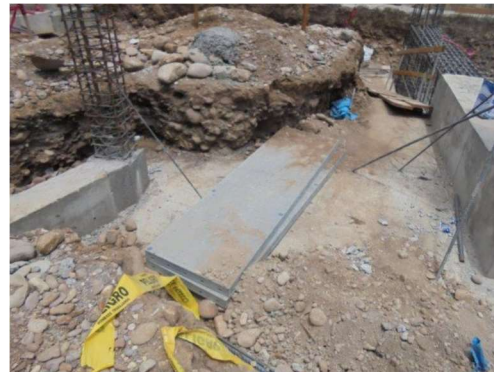
Figure 2.10. Surplus formwork partially buried on site
