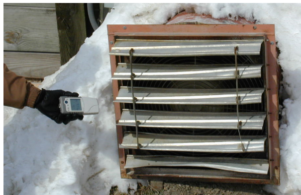
Figure 2. Handheld sensor measuring CO 2 concentration in the exhaust air stream of a fan on a ground pile.
