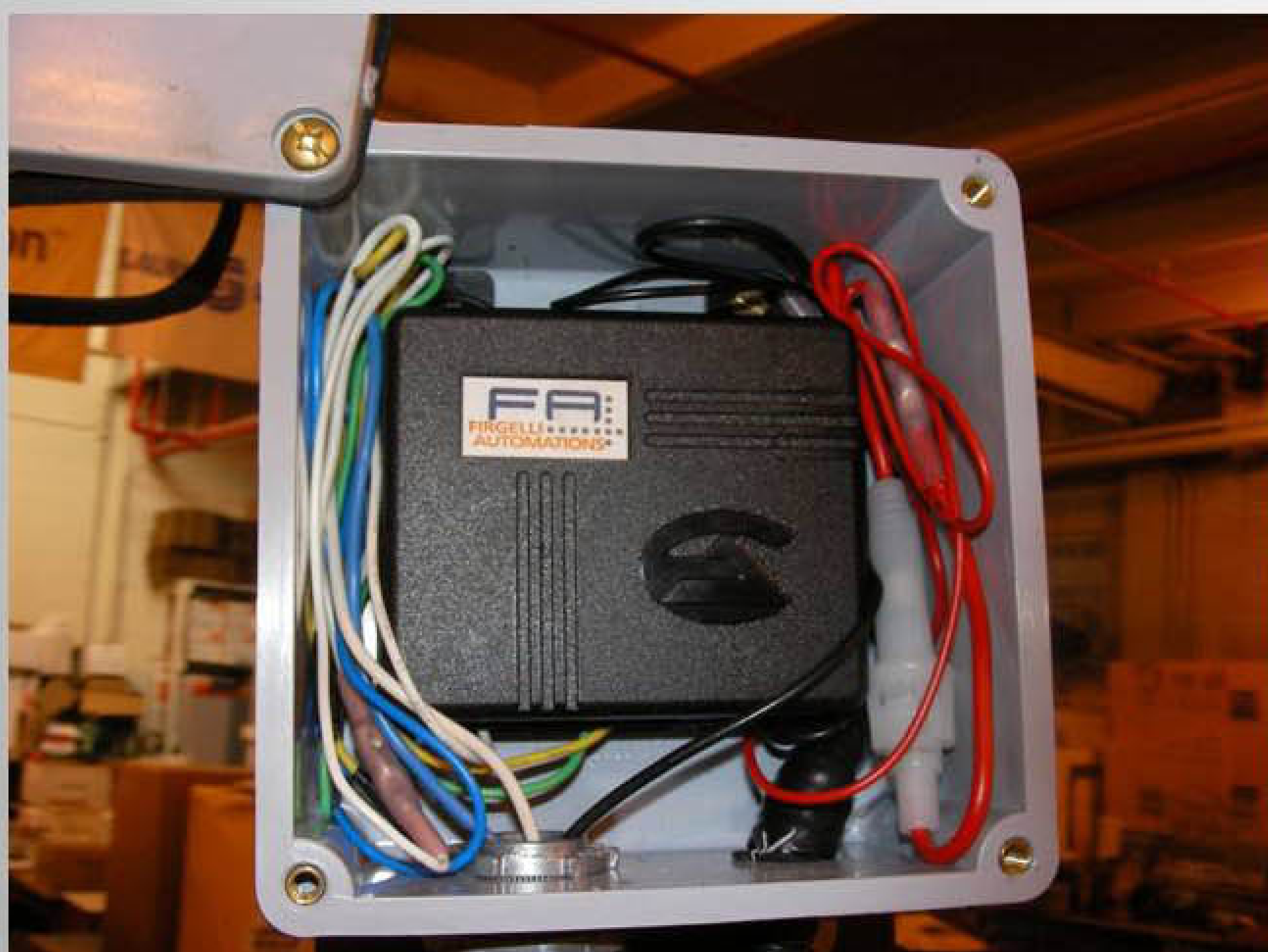
Remote Receiver and wiring in weatherproof box
