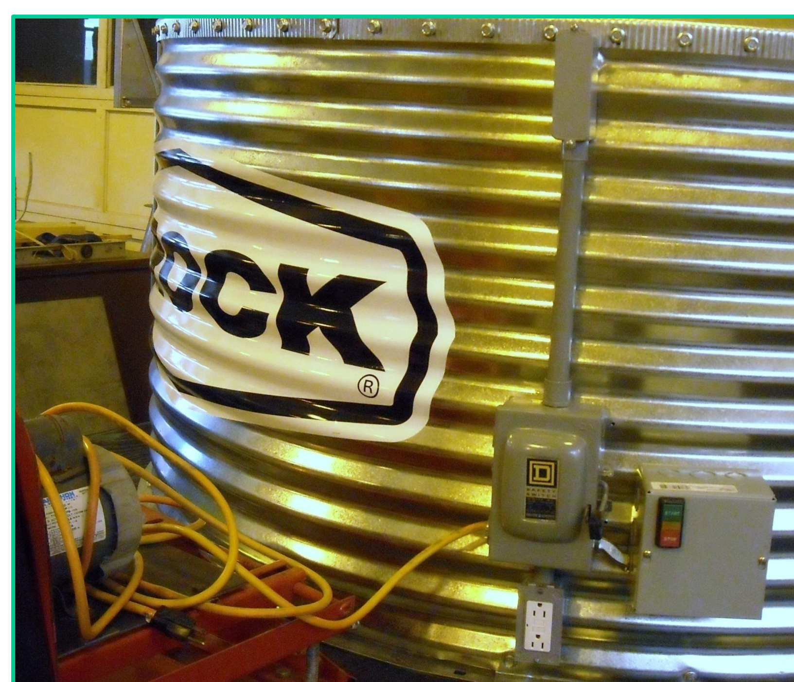
Electrical box, motor and contactor reset switch
