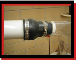
Pipe Reducer (Manifold to Cyclone Filter)
