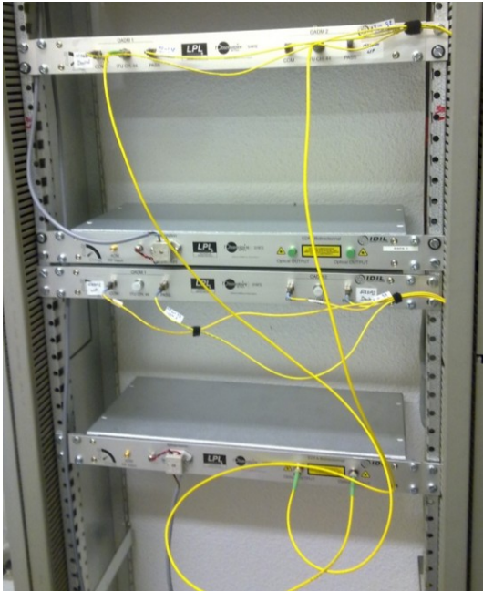
Figure 2. OADMs and bidirectional amplifiers inside the shelter of Condé sur Marne
